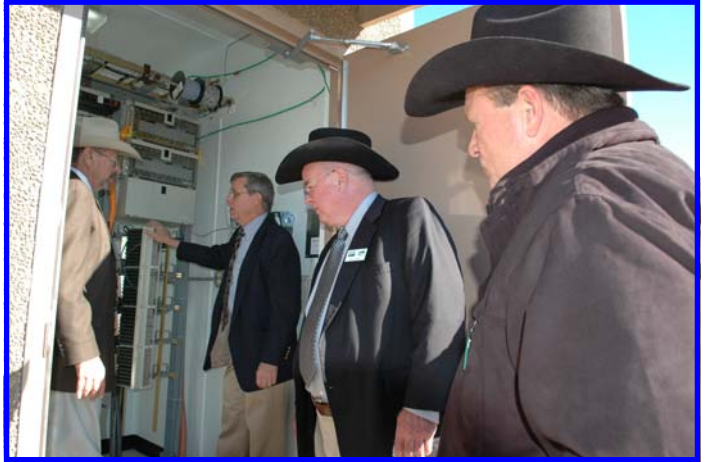
Steve Guest with Central Cellular provides technical information about the company's new broadband system and fiber optic setup to Area Directors Tom Barber, Jerry Tucker, and Jerry Efurud.
